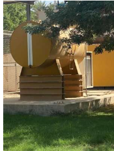
Tank for water treatment
