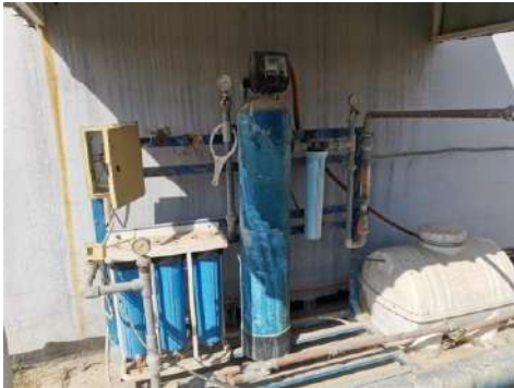
Filters for water treatment
