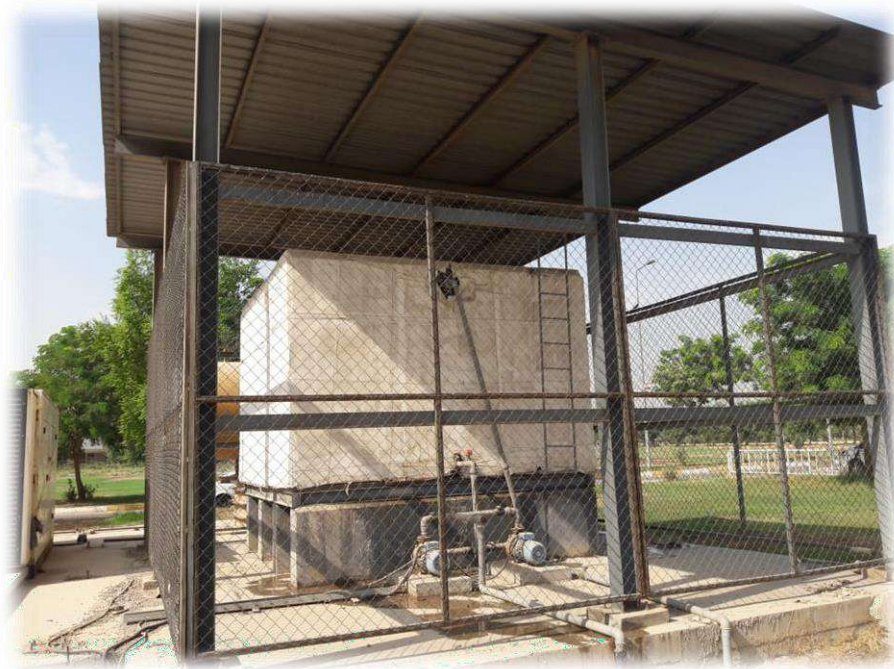
Tank to store rainwater
